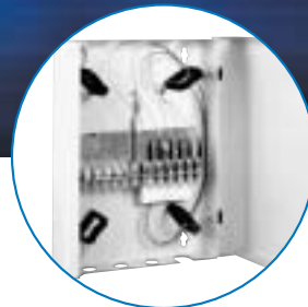
installed: 2 splice cassettes, 1 patch panel (12 ports) 1 patch panel (pre-wired with 12 ports)
